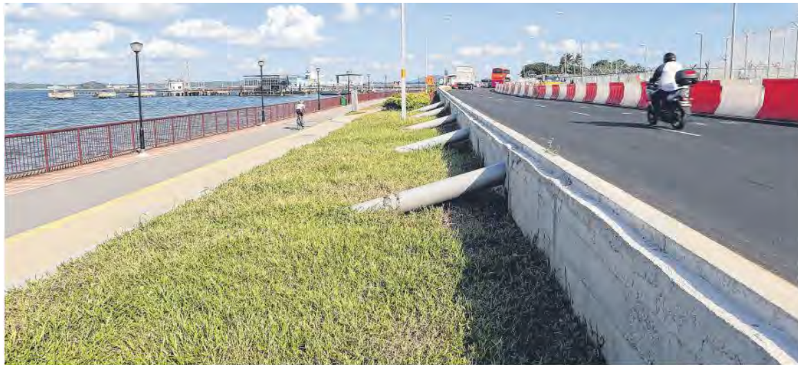
The coastal Nicoll Drive in Changi was raised by up to 0.8m last year, in anticipation of rising sea levels brought on by climate change. It was Singapore's first road-raising project of its kind. ST FILE PHOTO
